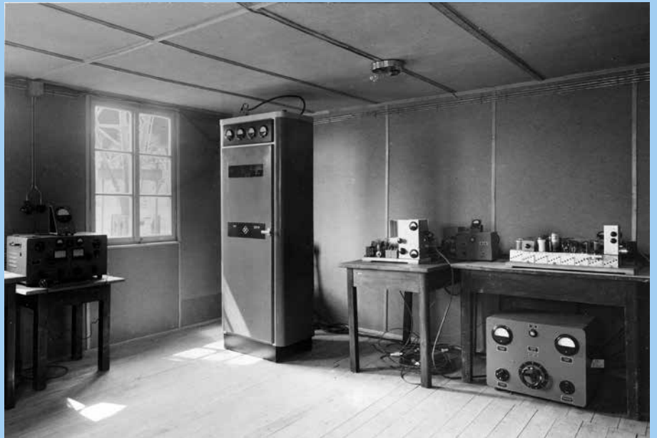
Europe's first commercial VHF FM transmitter went into operation on February 28, 1949. The supplier was Rohde&Schwarz. This photo was taken in the 16 m 2 wooden structure operated by the Bavarian Broadcasting Corporation at the foot of the antenna tower in Munich-Freimann.
